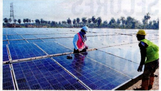
Tenaga Nasional Bhd's first large-scale solar project in Kuala Langat, Selangor, has a generation capacity of 50MW with DC install capacity of 78MWp.
